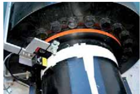
Fig. 1: Measurement of torque, speed and angle of rotation on a wind energy converter's main shaft. Photo: Frank Ryll
