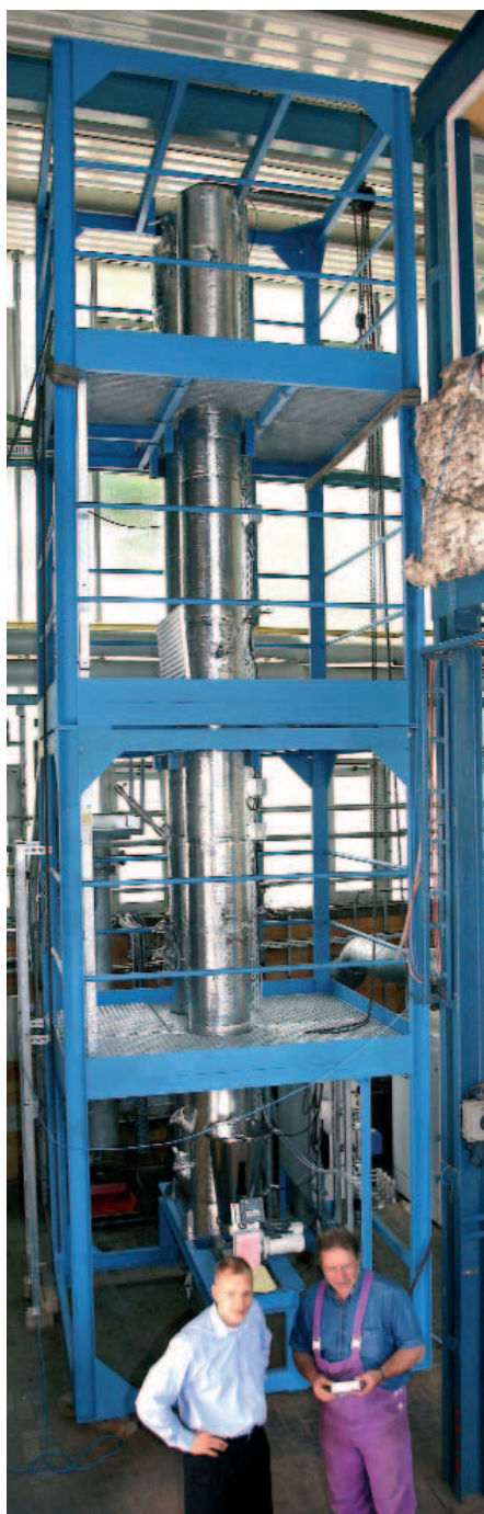
Figure: Erection of the circulating fluidized bed combustion plant or CFBC in Vietnam.
