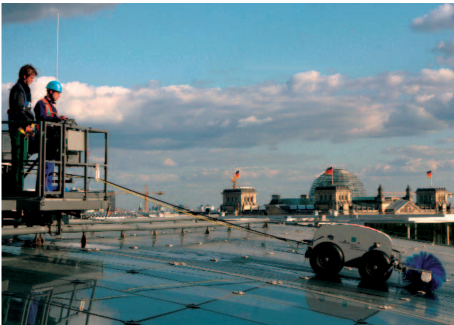
Figure 2: Performance tests on the roof of Berlin Central Train Station. The client has already presented the unit's at work in a television reportage.
